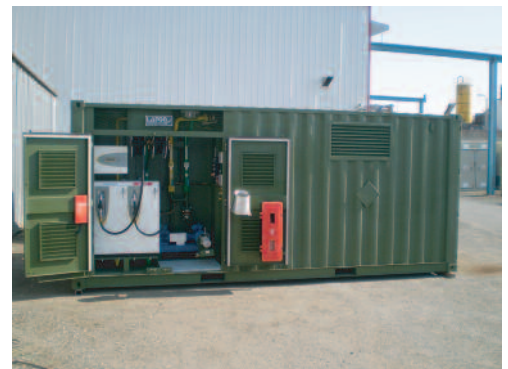
Station conteneur Mobiltank
